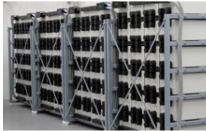
Energy Storage System
